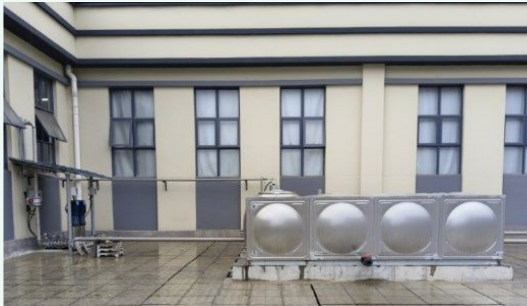
Huizhou Highpower Production Waste Water Recovery Project
