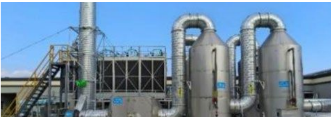
Air emission treatment facilities
