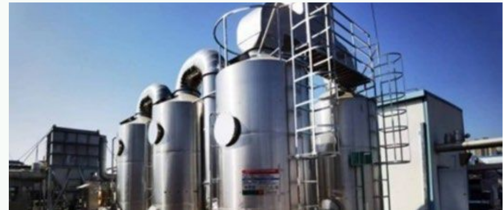
Reconstruction of NMP air emission treatment equipment
