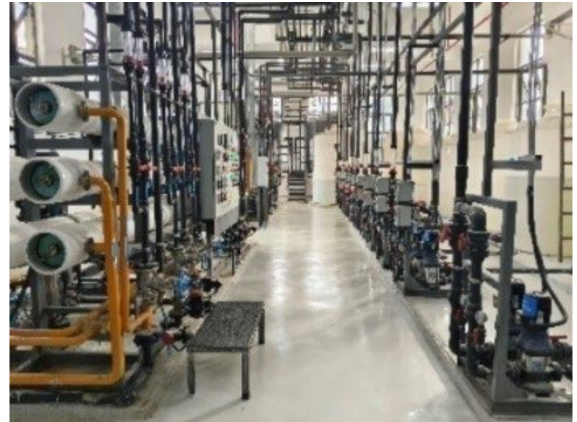
Wastewater treatment station
